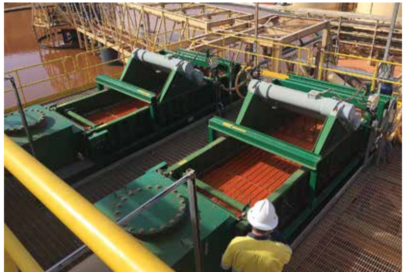
Derrick W56 Trash Screen removing carbon at 600 microns
