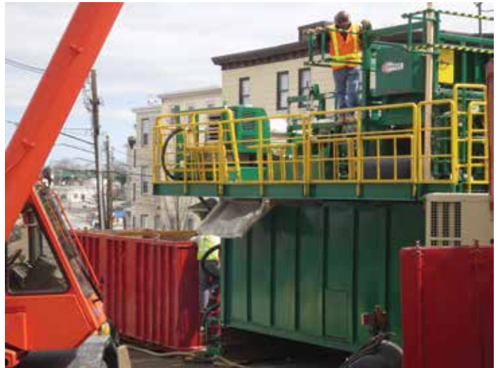
Derrick Modular Slurry Separation Plant in operation
